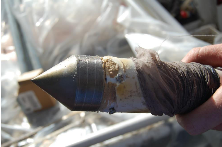
Figure 38. A Broken and Cracked Belled-End
