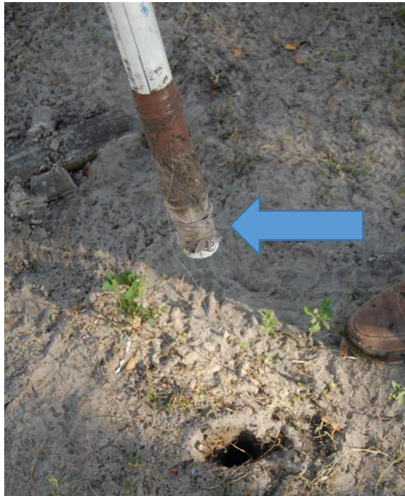
Figure 34. Break in Pipe for Well #3
