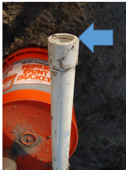
Figure 37. Failed PVC Adapter on Well #5
