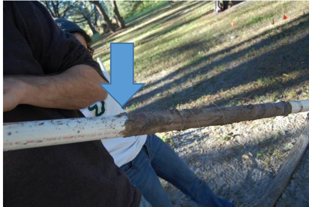
Figure 36. Failed Screen on Well #5
