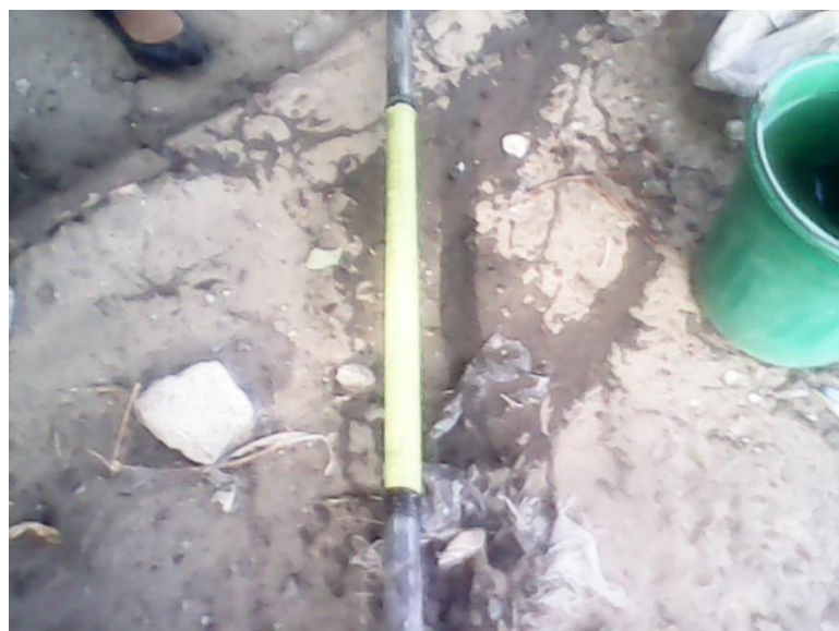
Figure 44. PVC pipe of Well #2 of the Madagascar System
