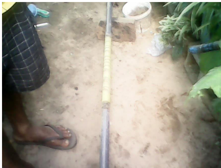
Figure 43. PVC pipe of Well #1 of the Madagascar System
