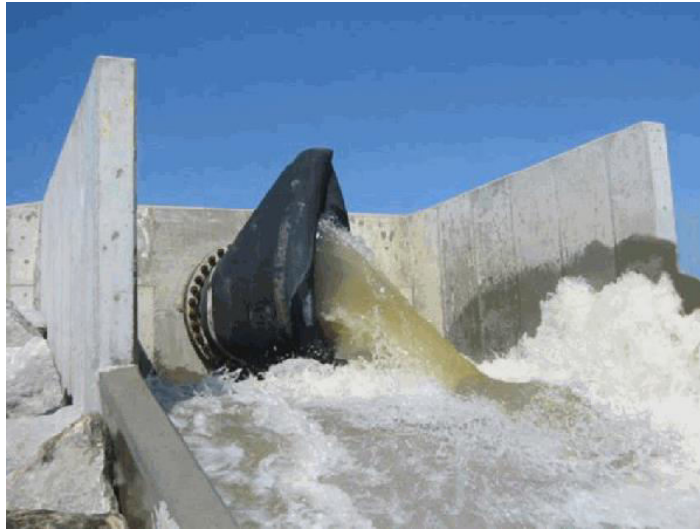
Figure 10. Duckbill valve serves as tide gate for outfall [16]
