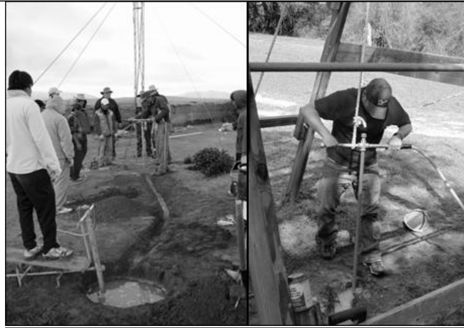
Figure 4: (a) EMAS percussion-jetting set-up, Bolivia [left]; (b) Test-drilling using percussion-jetting at the University of South Florida GeoPark [right] (M. MacCarthy)
