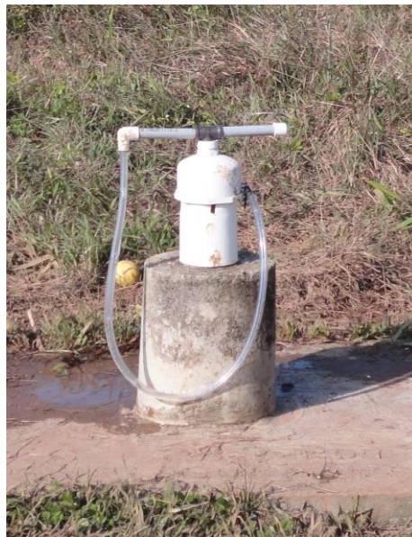
Figure 11: EMAS Pump Installed by the Healing Fund
